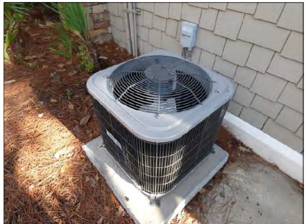
Ranger Station HVAC
