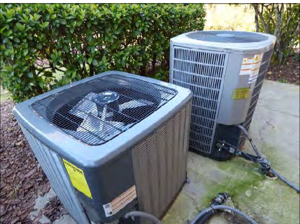
Nature Center HVAC
