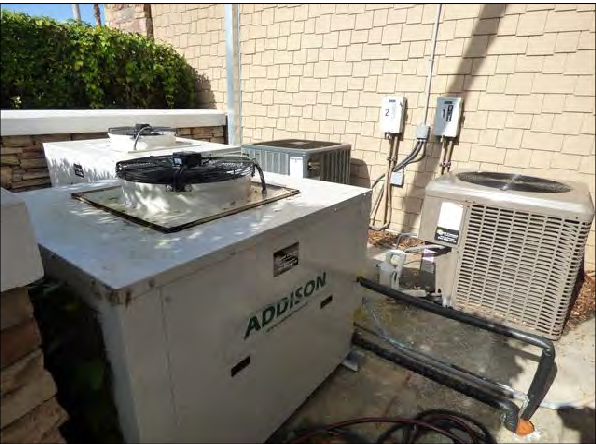
Fitness Center HVAC
