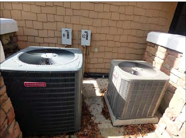
Activity Center HVAC
